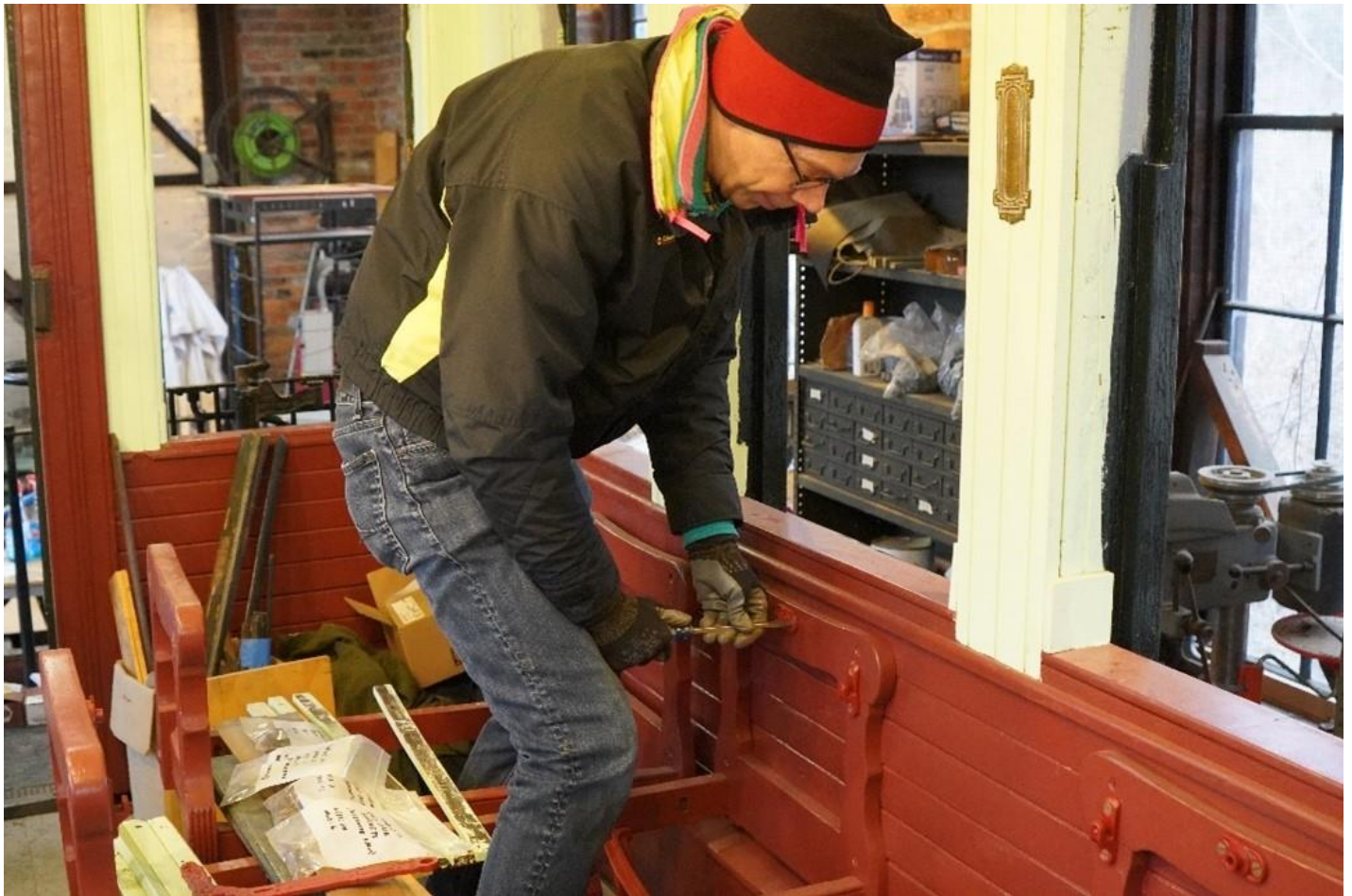
Eric Knepp installs hardware on the wooden seat frames in Combine 14. – Al Gallo photo
