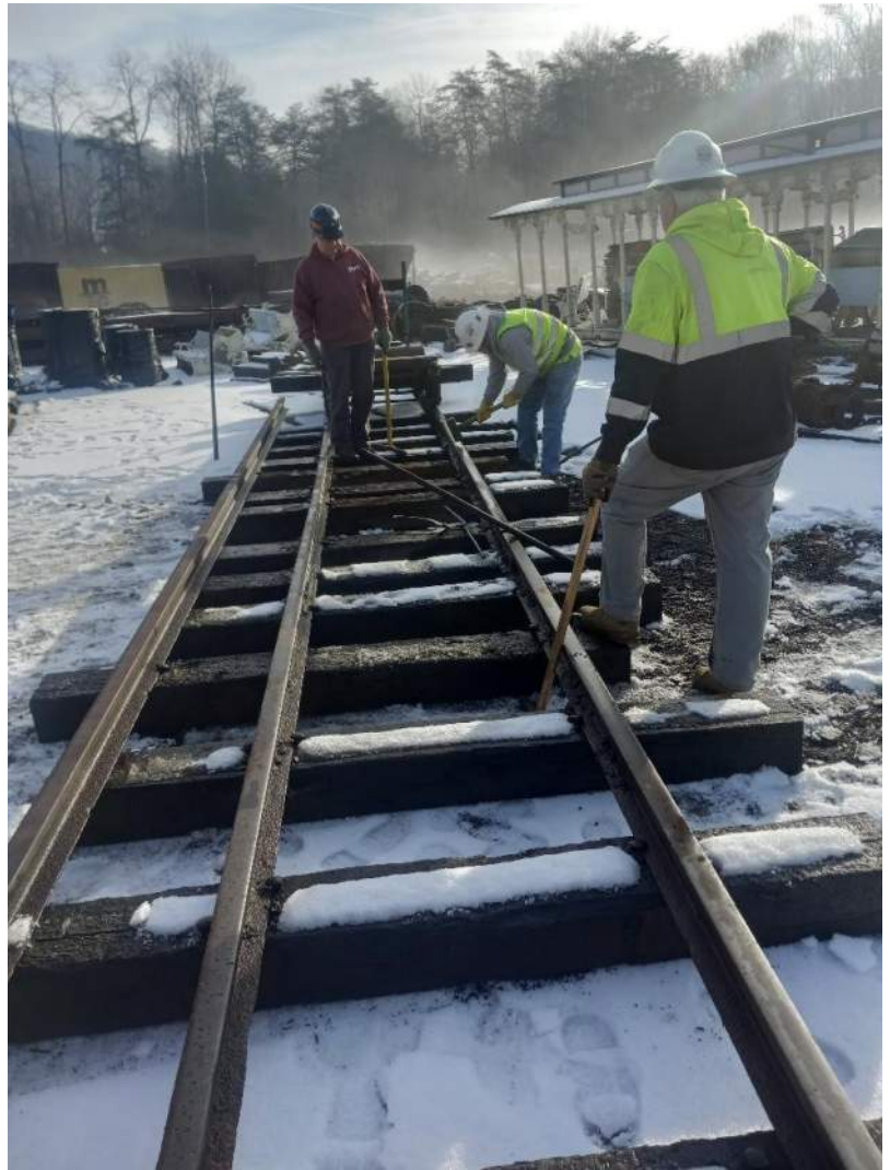
The track crew assembles a dual gauge track panel to be used as a work platform for regauging the new tie inserter on December 17. – Gene Tucker photo
