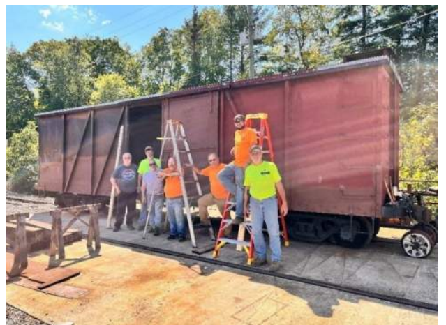
Boxcar 174 and crew after re-installation of the second sliding door. – Dave Bulman photo
