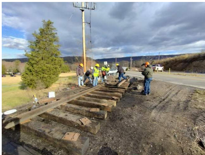
Above: On December 3, a cold track crew makes preparations to connect the main line rails to the rails in the Pogue Road crossing. – Gene Tucker photo
