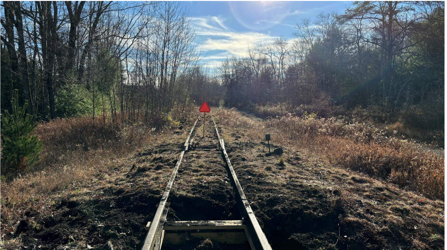
The new southern end of usable track for speeders and railbikes just north of Woodvale, as established on November 9. – Sam Painter photo
