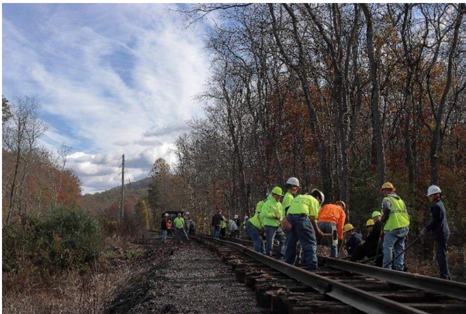
The combined forces of the EBT Foundation track crew, the FEBT track crew, and FEBT's Young Easties work at installing track between the McCoy Road and Pogue Road (PA 994) grade crossings on October 26, 2024. This work is part of the March to Saltillo. – Chris McCann photo
