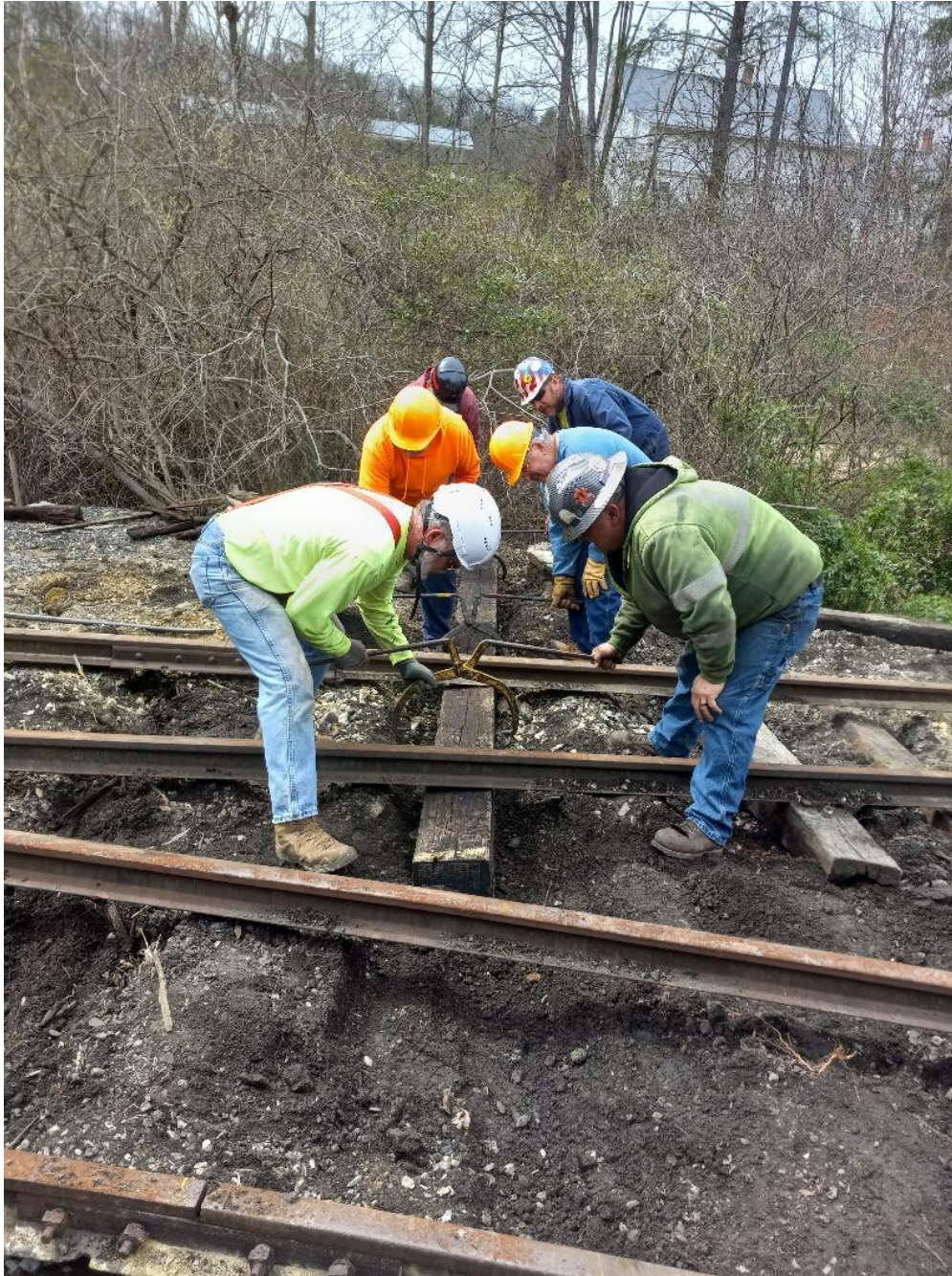
FEBT Track Crew members replace switch timbers in the Paint Shop lead track. – Gene Tucker photo
