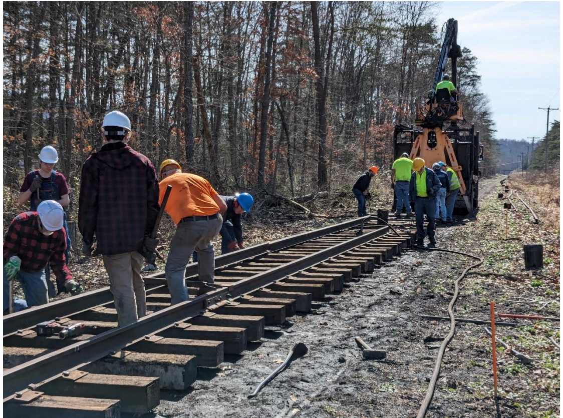
East Broad Top track forces gauge the rails installed south of the Maddensville Pike grade crossing on March 12 th . – Al Gallo photo
