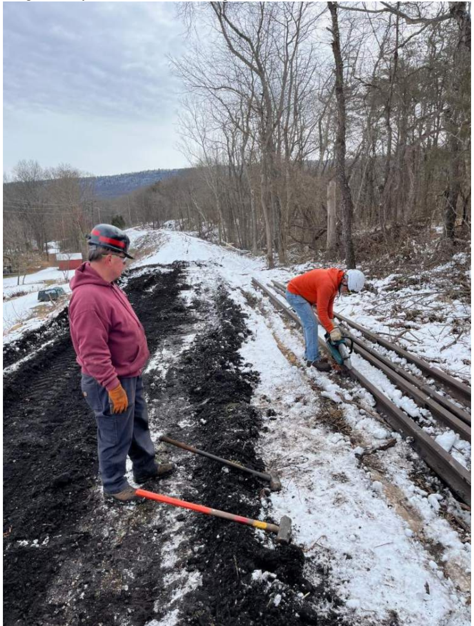
Bolts are removed from the rails on the south face of Jordan Summit. The rails have been pushed to the side to allow for regrading of the roadbed. New bolts will be installed when the rails are reassembled. – Jack Fornadley photo
