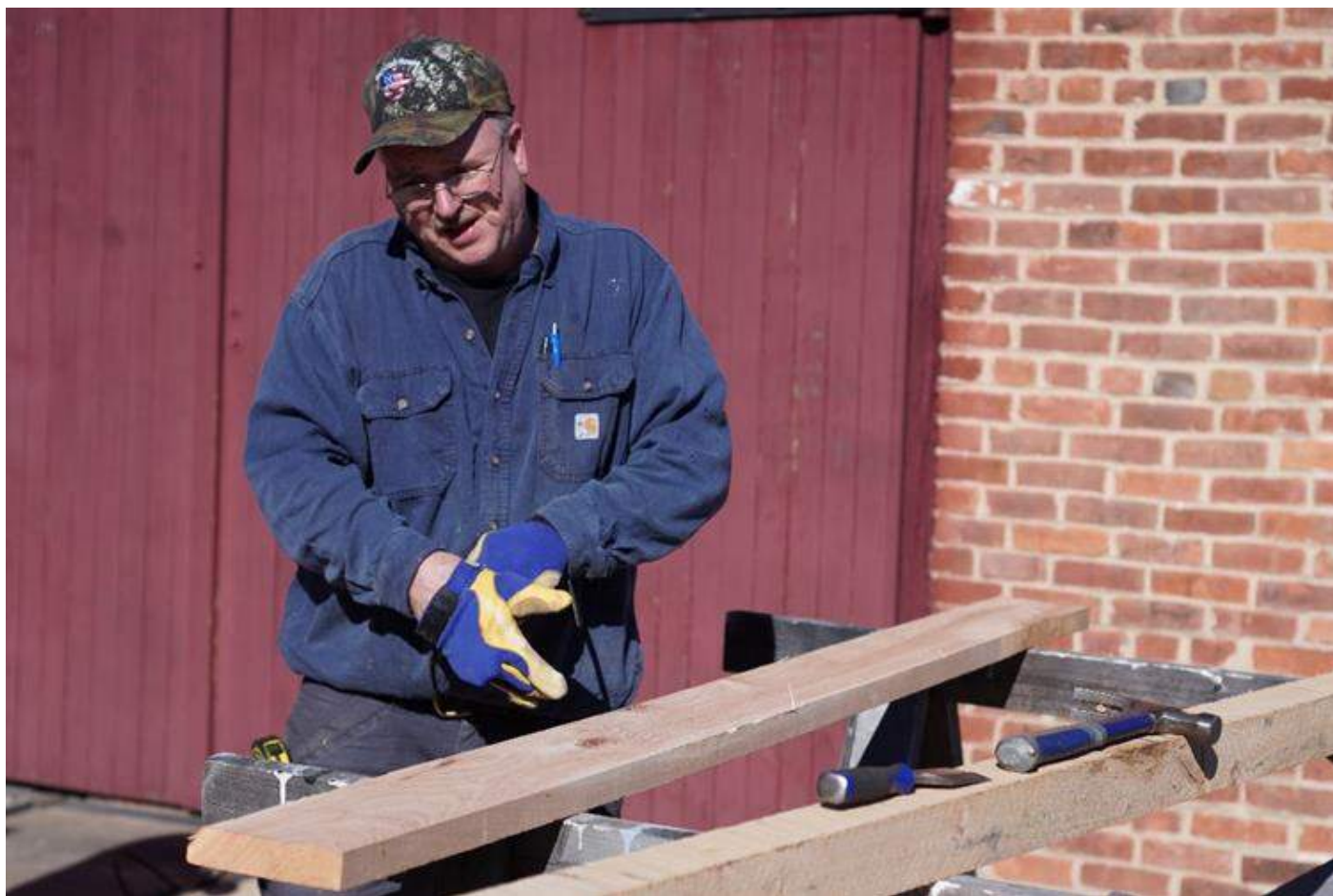
Lamar Tyson prepares oak floorboards for installation in Boxcar 174. – Al Gallo photo
