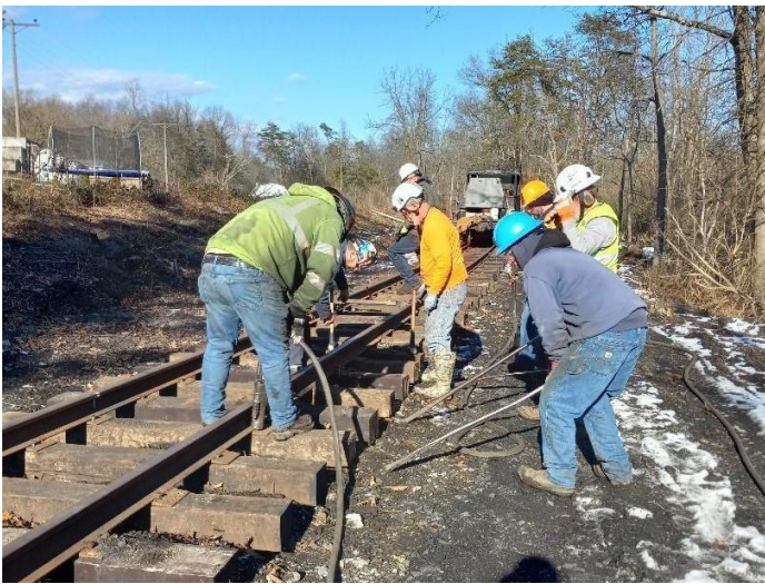
FEBT track crew installs ties on the mainline south of Rockhill approaching Rt. 475. – Gene Tucker photo
