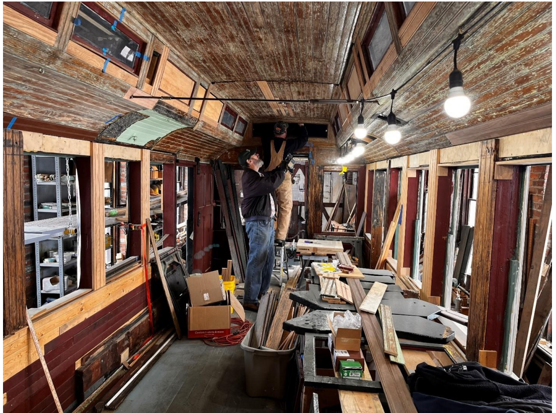
Right: Mark Reese and Lamar Tyson work on final assembly of the baggage section of Combine 14. – Dave Bulman photo Below: Tom Perman, Jill Confair, and Craig Confair with the first new door frame for the north end of the Car Shop. – Dave Bulman photo
