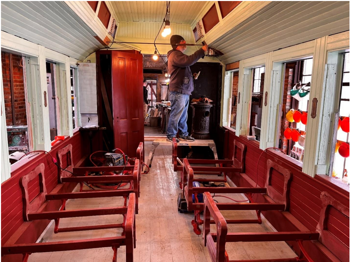
Dave Ebright works on finishing touches in the passenger compartment of Combine 14. – Dave Bulman photo.
