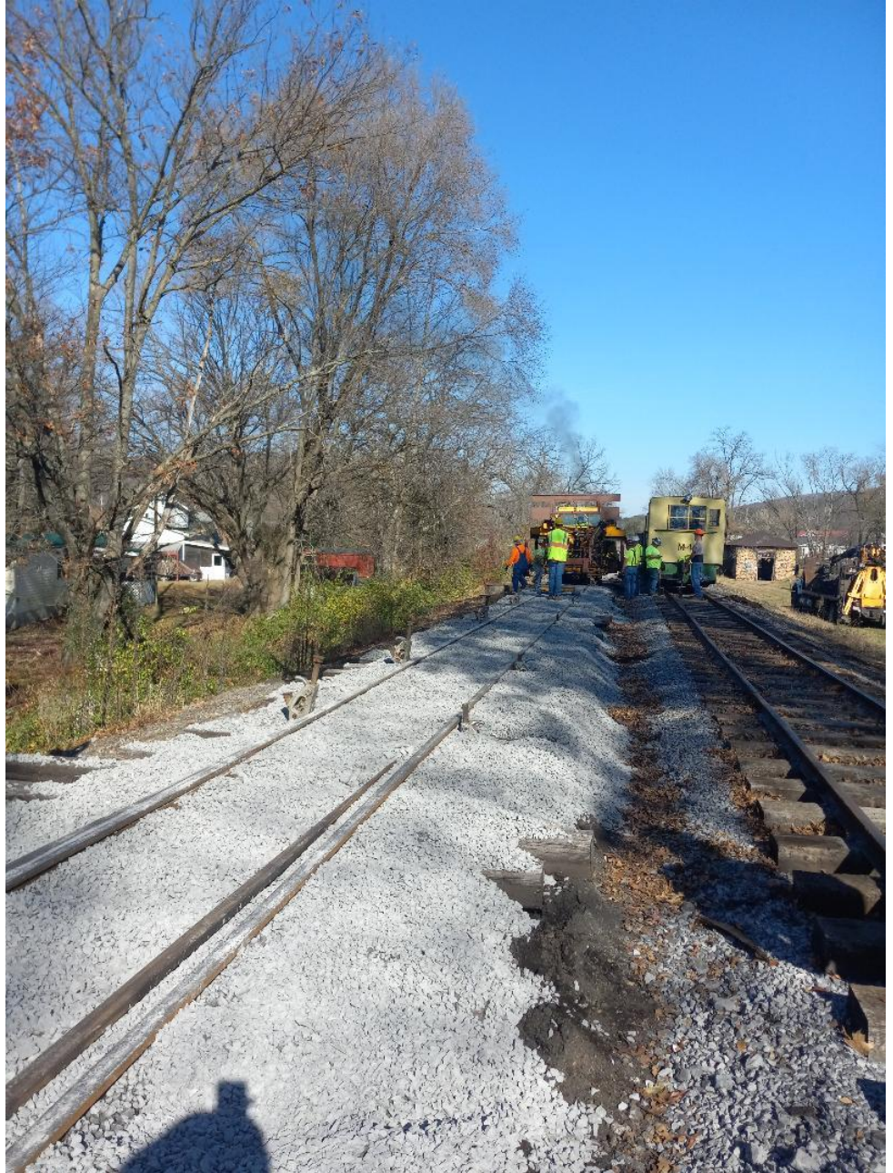
FEBT Track Crew members assist EBTF personnel with maintenance on Tracks 2 and 3 at the north end of the Rockhill Yard. – Gene Tucker photo
