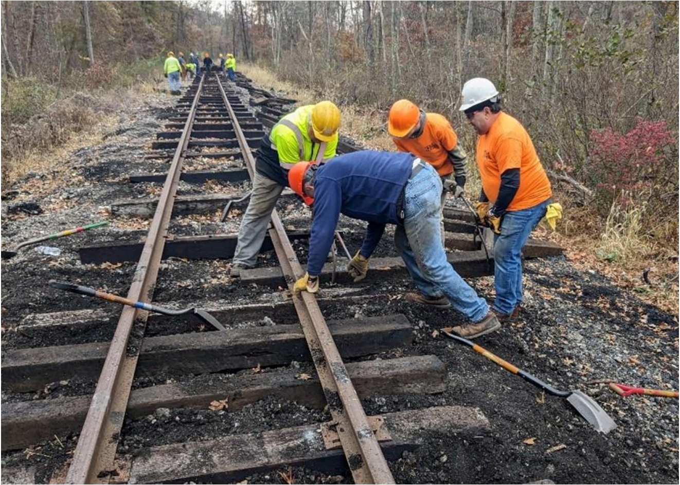
FEBT Track Crew members insert ties into the main line between Oddfellows Cemetery Road and Maddenville Pike grade crossings. – Al Gallo photo
