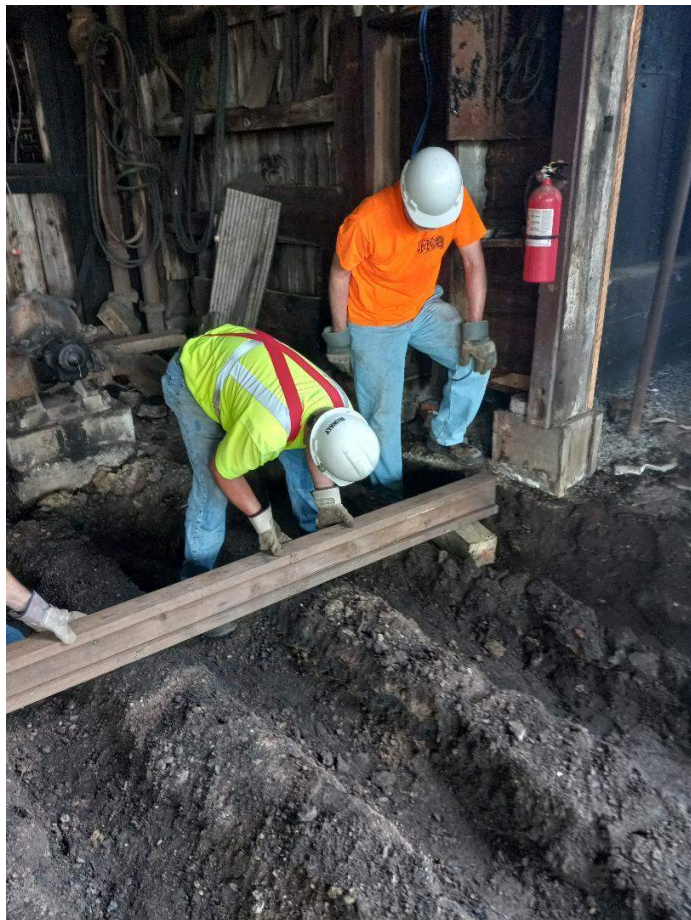
John Quinn and Tim Schindele work together to verify the cribs in the Car Shop have been dug to the current depth on August 19 th . – Gene Tucker photo
