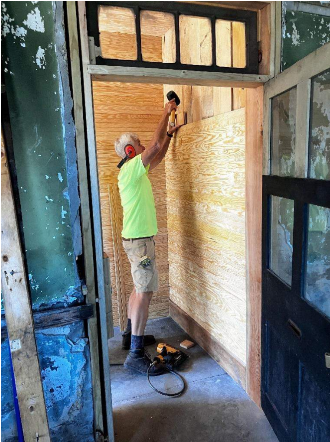
The window crew continued rebuilding and installing multiple window sashes, installed the final window in the Car Shop south wall, and painted window trim on the Storehouse.
