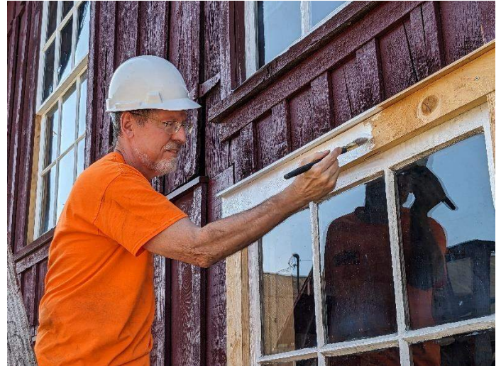
Above: Doug Linebaugh paints the recently-installed Storehouse window frames during the August work session. – Eric Knepp photo
