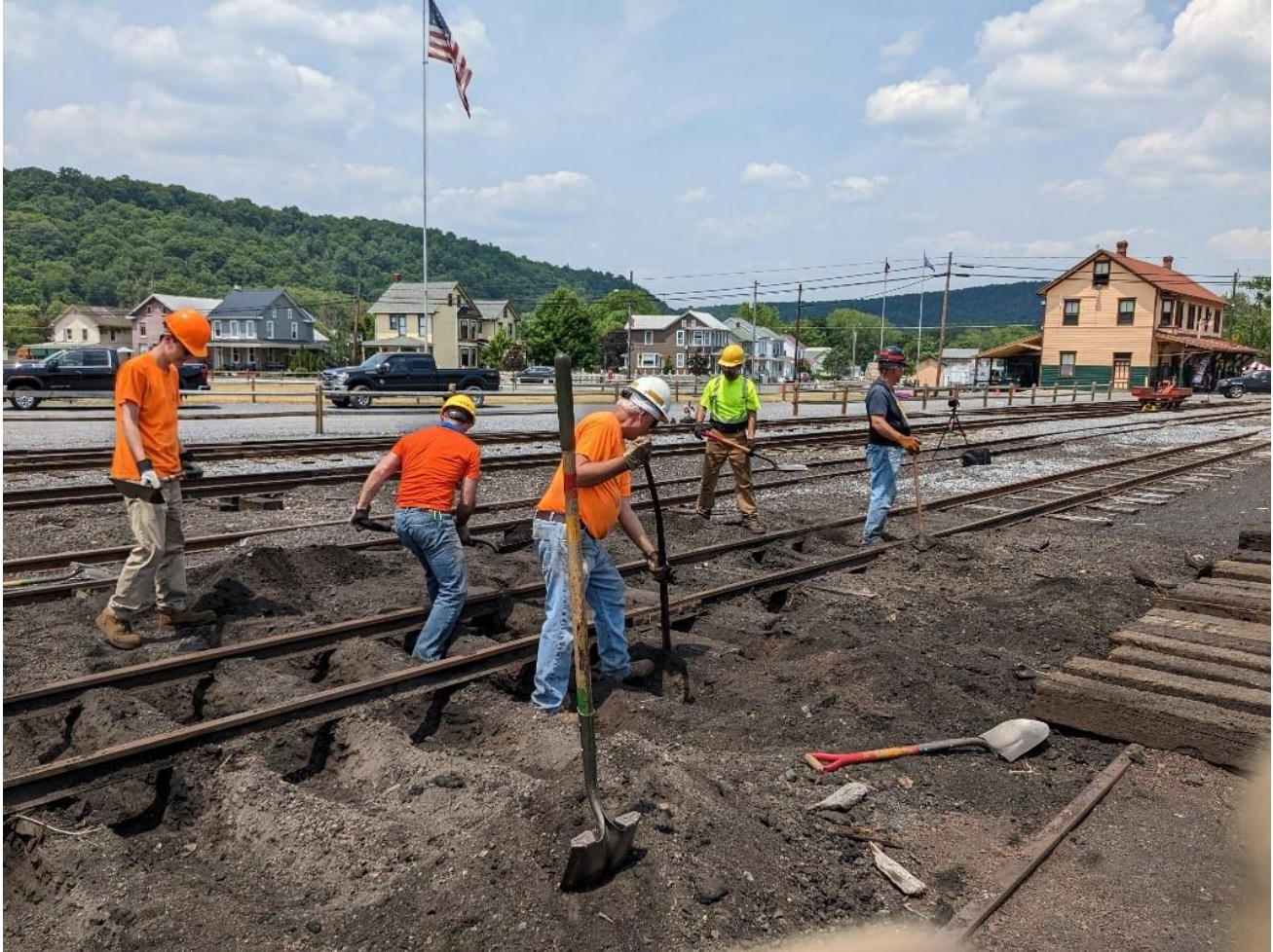
Jackson Ganser, Tim Schindele, Larry Fuchs, Chris Wenger and Daniel Lane work to install new ties on Track 4 near Meadow Street. – Al Gallo photo
