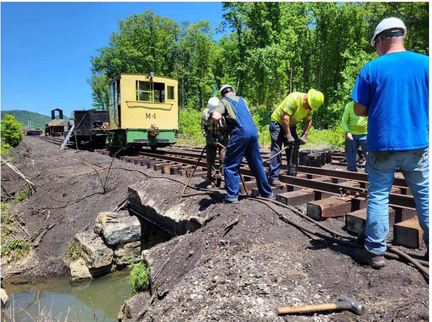
The FEBT March to Saltillo is in progress, as track crew members Gene Tucker, Sam Painter, Chris Letcher, Todd Johnson, Tom Perman, and Don Bayer spike up new ties in the main line to the south of the coal dock during the FEBT Spring Work Week. – Andy Van Scyoc photo
