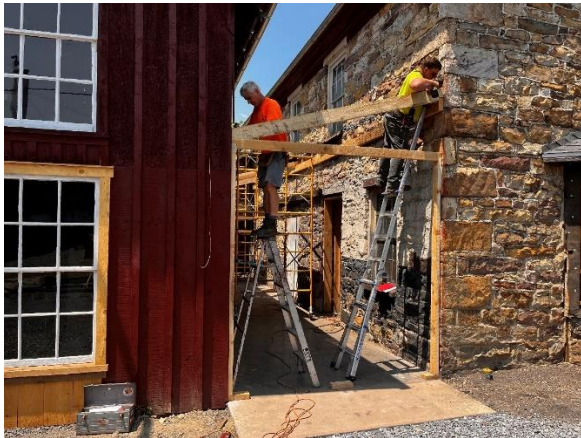
Left: Craig Confair and James Roslund install the first new roof rafter of the lean-to. – Dave Bulman photo
