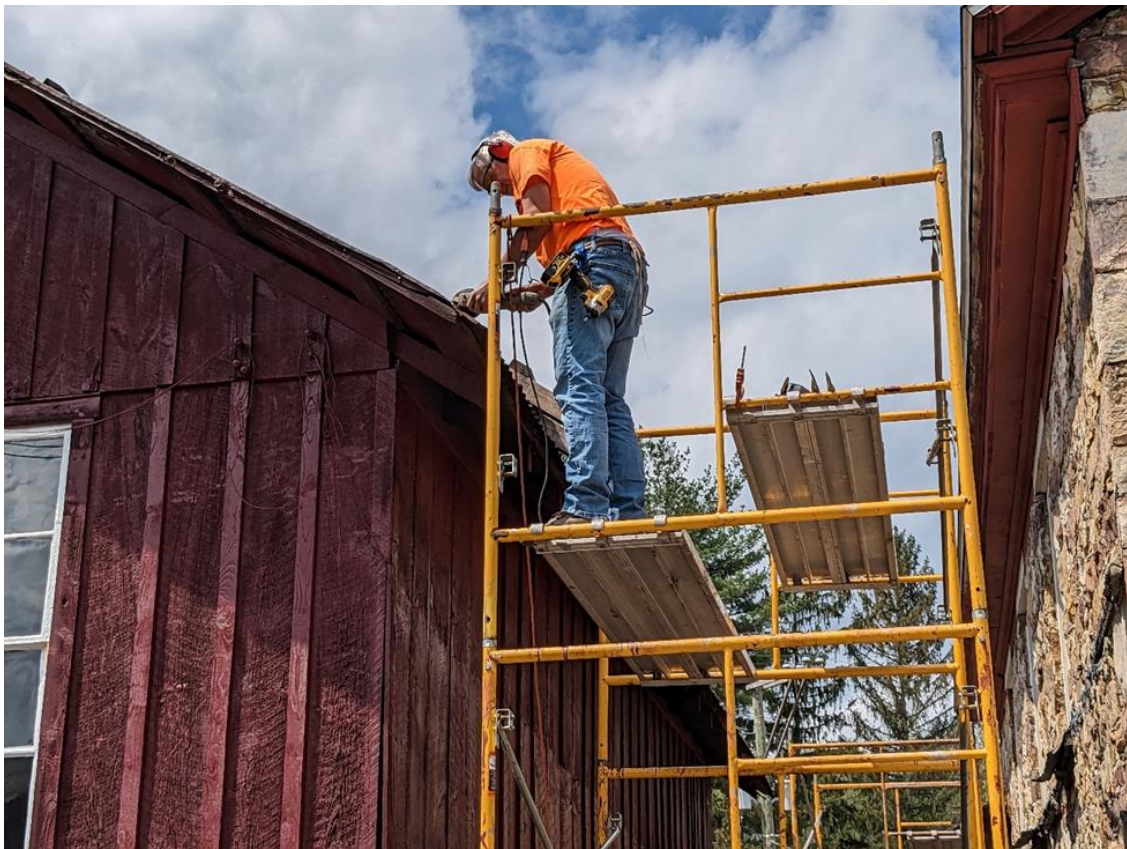
Craig Confair makes repairs to the Storehouse roof prior to the lean-to being reinstalled during the upcoming Spring Work Week in May. – Al Gallo photo
