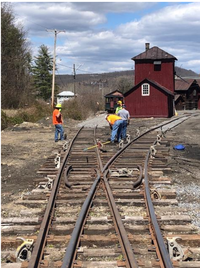
During a mid-week trackwork session on April 4 th , the crew levels and regauges the Paint Shop and Roundhouse lead tracks on the western edge of the Rockhill yard. – Gene Tucker photo
