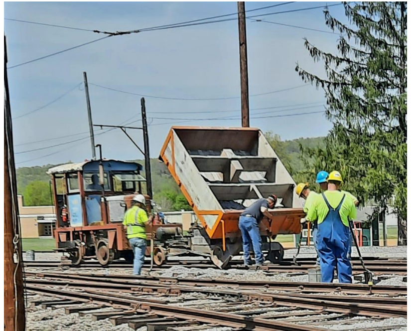
Like a good neighbor, the FEBT Track Crew is there, assisting the Rockhill Trolley Museum in the Car Barn 2 yard area with tie replacement during the week of April 17 th . – Gene Tucker photo
