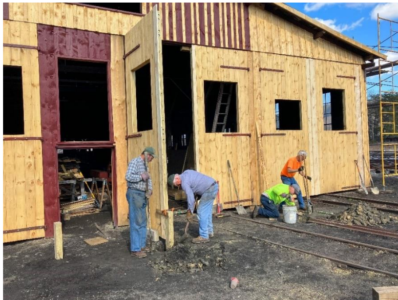
Mark Reese and Larry Fuchs work on setting a door stop while Tom Perman and Craig Confair work on a hole to set another door stop at the south end of the Car Shop, March 5, 2023. – Eric Knepp photo
