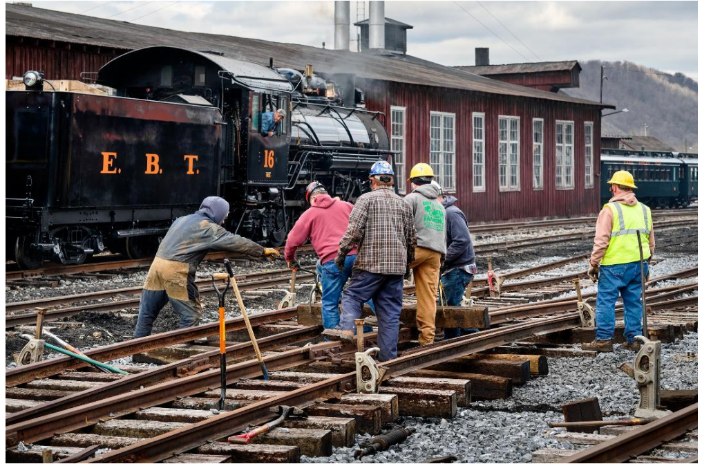
EBT Master Mechanic Dave Domitrovich stops No. 16 to watch the FEBT Track Crew of Gordon Ley, Daniel Lane, Henry Long, Chris Wenger, Ryan Rimshaw, and Gene Tucker install new ties in Tracks 4 and 5 at the south end of the Rockhill Yard on February 10 th . Additional opportunities to see steam engines in action is one of the benefits of volunteering. – Matthew Malkiewicz photo
