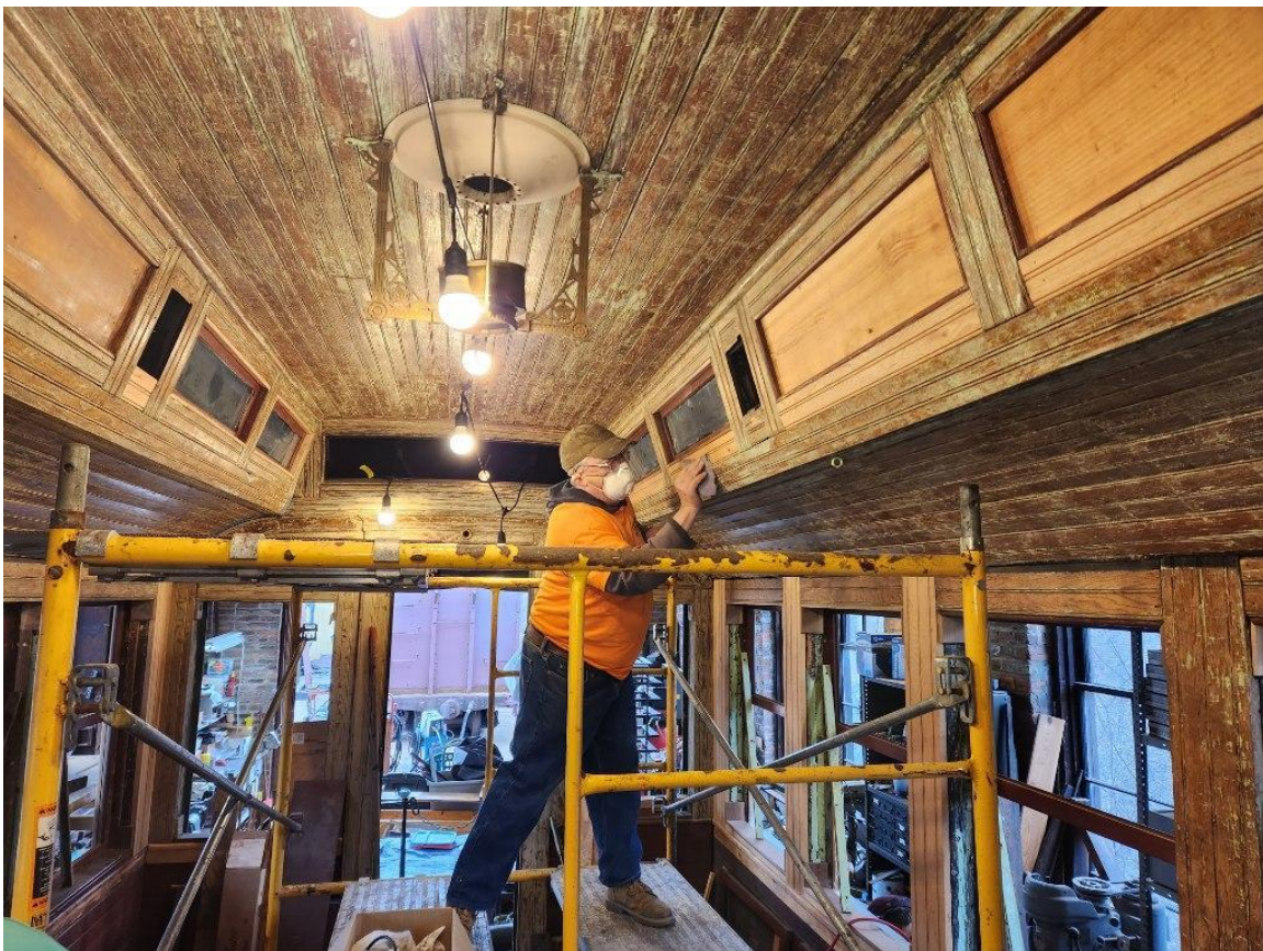
Thomas Faust sands the woodwork on the interior of Combine 14 during the January 2023 Rockhill Work Session. – David Ebright photo
